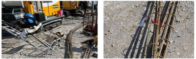
Damaged excavator and reinforcement cage Reinforcement cage with rings all around
